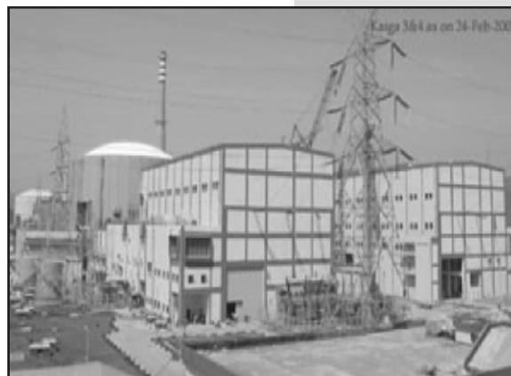
Kaiga Atomic Power Project 3 & 4
