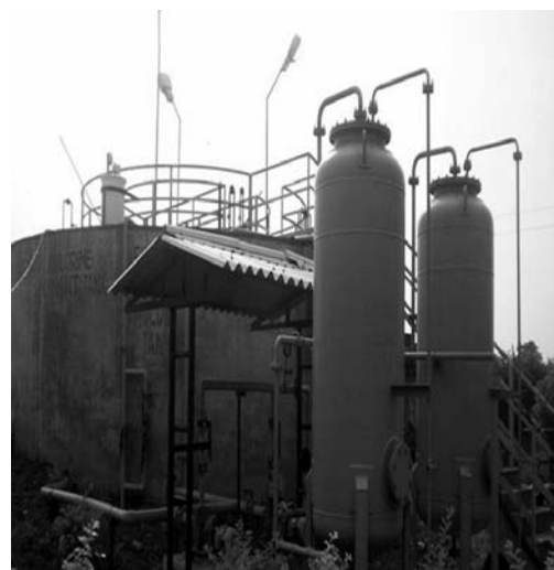
ETP at Himalayan Institute of Hospital Trust.
